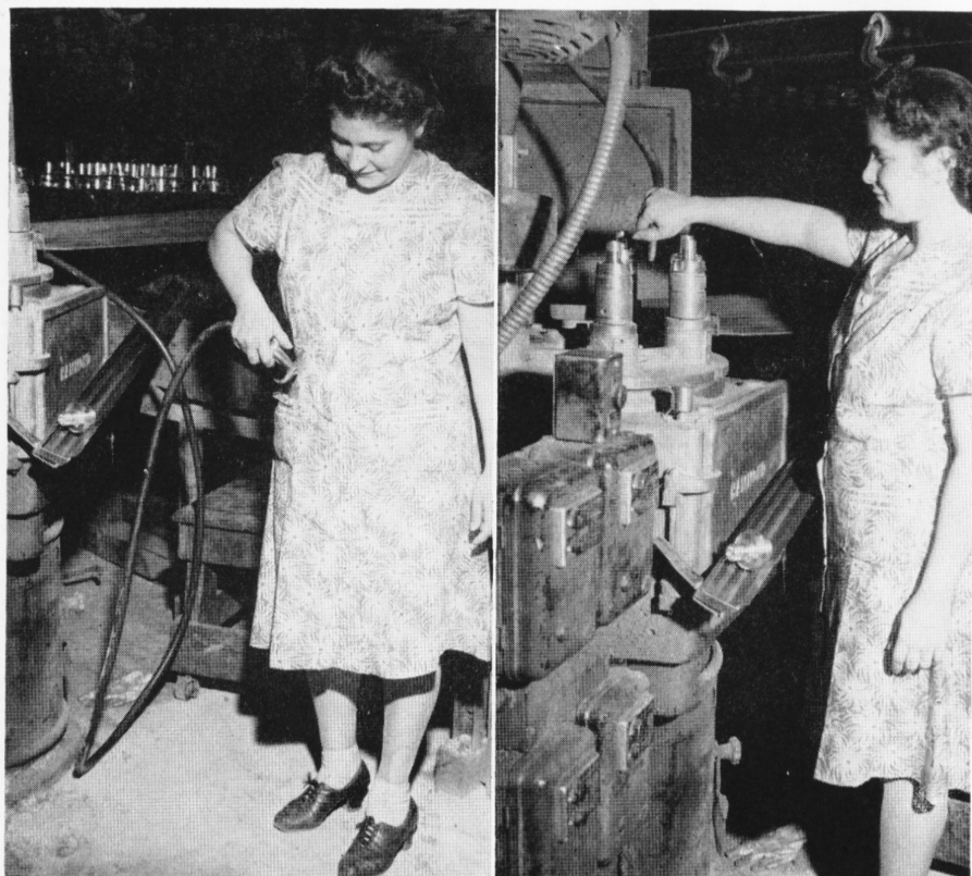
The picture on the left shows an unnecessarily long hose, which was sometimes misused for cleaning clothes. Carmella DeSantis is holding, in the picture on the right, the same hose which has been shortened to prevent misuse by persons unaware of the dangers involved. The hose is still long enough to be used on the machine.
